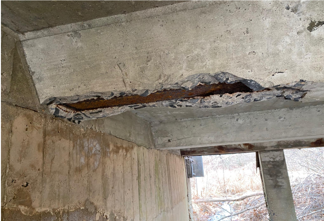
Typical Steel Girder encased in Concrete Spalling
