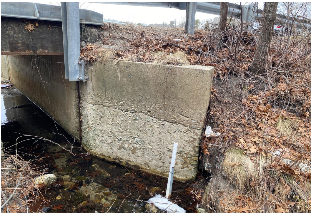
Typical Scaling on Abutments and Wingwall
